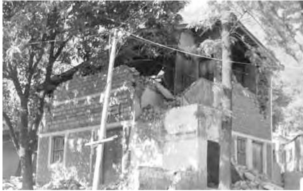
Figure 7.1 : A Damaged Building Due to an Earthquake
