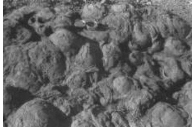
Fig.6.4 : Exfoliation (Flaking) and granular disintegration
